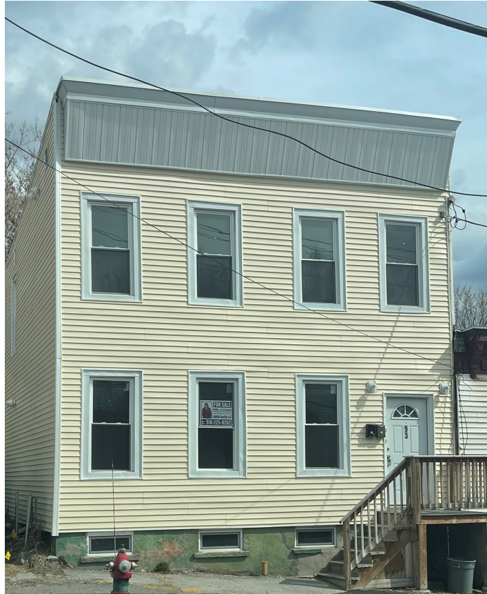
Rehabilitation of a vacant property acquired from the Albany County Land Bank completed in Albany, New York.
